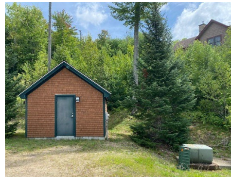
This pump station was built during the Cascade Ridge Subdivision development in 2005. The station contains two pumps used to boost water pressure to several properties located on Bean Bender Road .
