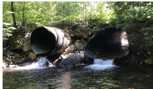
Perched Culverts, Chickenboro Brook, Thornton (Source: NH Geological Survey, NH Aquatic Restoration Mapper)
